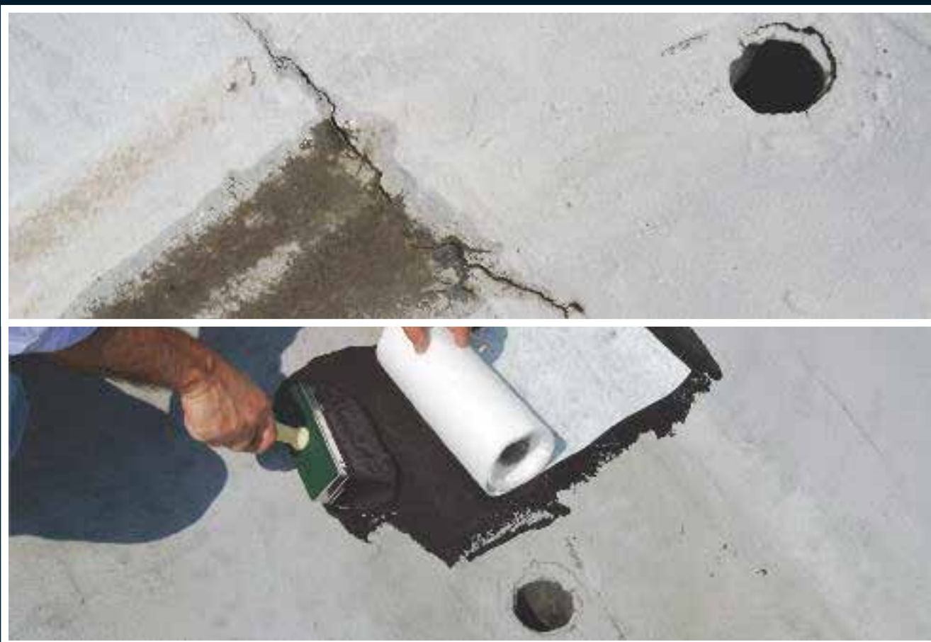
To repair and waterproof cracks (in the photograph: repairing a crack on a bituminous membrane near a roof drain) applying ElastiK and Supporto Antifessura
