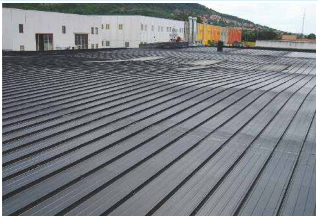
How the metal roof looked like after treating it with two coats of ElastiK applied 48 hours apart (spray-painting, 1 kg/m 2 )
