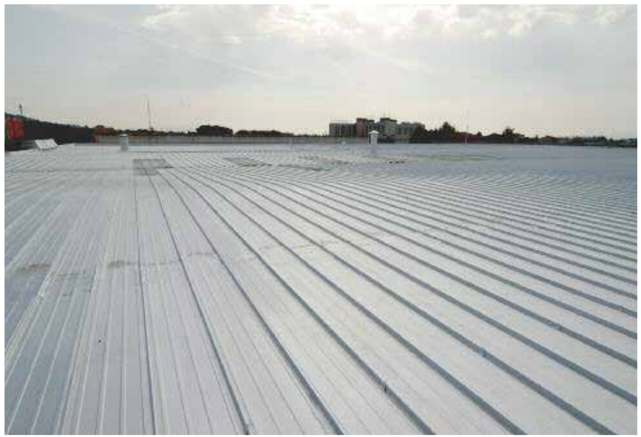
How the metal roofs looked like after treating it with one coat of aluminium paint like Allumisol 12/14 , applied 20 days after the second coat of ElastiK (spray-painting, 200 g/m 2 )
